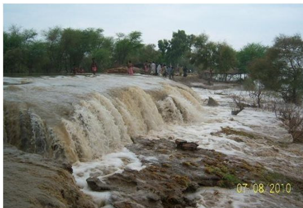
View of splitting Toori dam in district Kashmore @ Kandhkot
